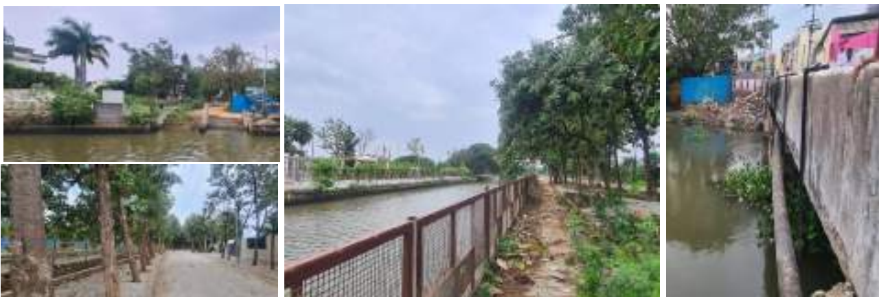
Figure 14-2: Present condition of Uyyakondan canal
