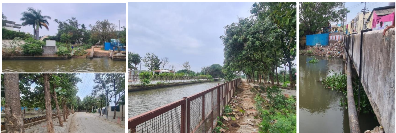
Figure 14-2: Present condition of Uyyakondan canal
